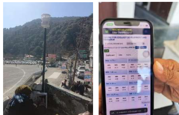
Fig. 19: AWS, installed in District Sports Academy building, Nainital.
